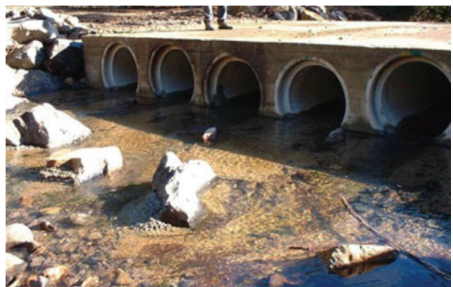
Multi-barrel circular culvert with culvert pipes at different levels to cater for high flows.
