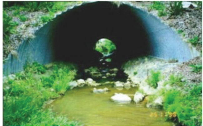
Good practice – single barrel arch culvert.
