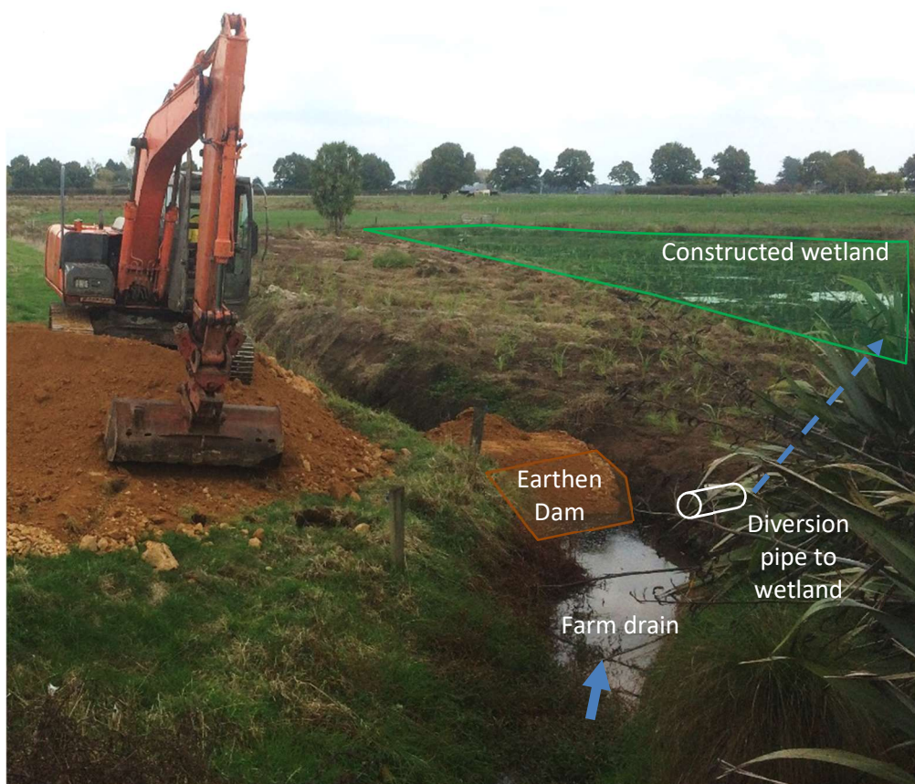
Figure 4: An off-stream wetland (in background) being connected to flow from a drain. An earthen dam (to be armoured with geotextile) has been constructed to block the existing drain. A pipe will be installed to divert the impounded water to the constructed wetland. Another pipe will be installed further downstream to feed this water back to the drain after passage through the wetland. Excess storm flows can still flow over the dam and down the drain.
