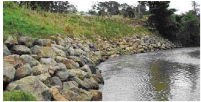
An example of an erosion control structure (rock rip rap).
