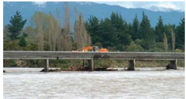
A multiple span road bridge during a high flow event. (Note the debris build-up on the bridge piers.)
