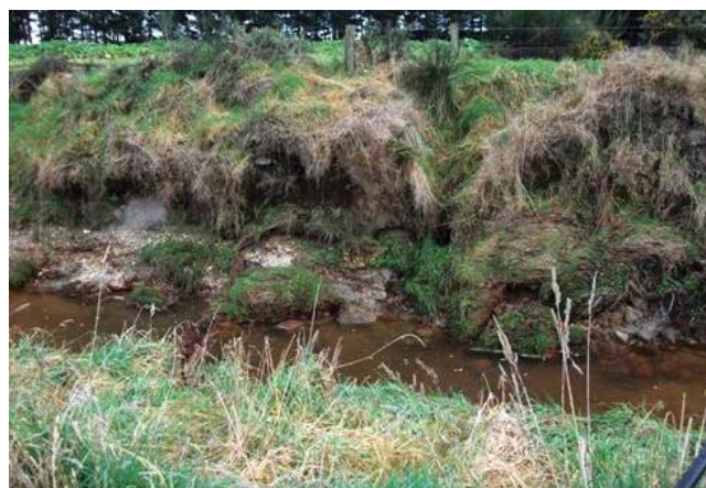
An example of moderate erosion.
