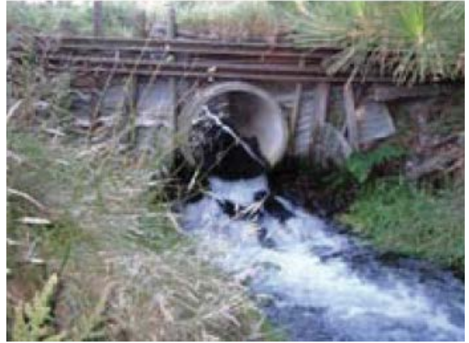
An example of a badly installed culvert, which has been placed too high above the stream bed, which increases erosion and prevents fish passage.
