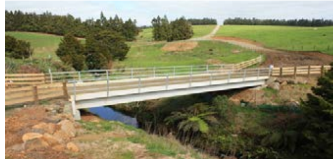
Good practice single span farm bridge. (Note that the footing of the bridge is well away from the water's edge at normal flow so that the natural river bank is retained under the bridge.)
