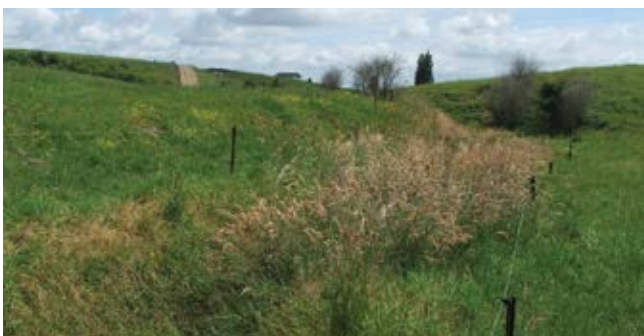
A weed-choked drain.
